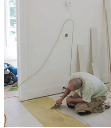
The flooring starts to go in and makes the house look so much lighter and more polished. It's exciting to see the space start to come to life.
