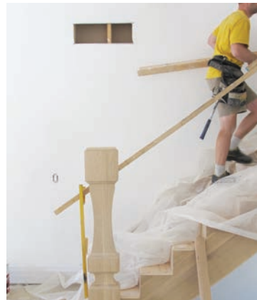
Stairworks/Flourish Design Elements custom-made the newel post. It gets oohs and aahs when it goes in and is the architectural moment we hoped for.
