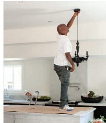
We originally tried these black candelabra-style lights over the island before choosing the stainless steel pendant lights that hang there now.
